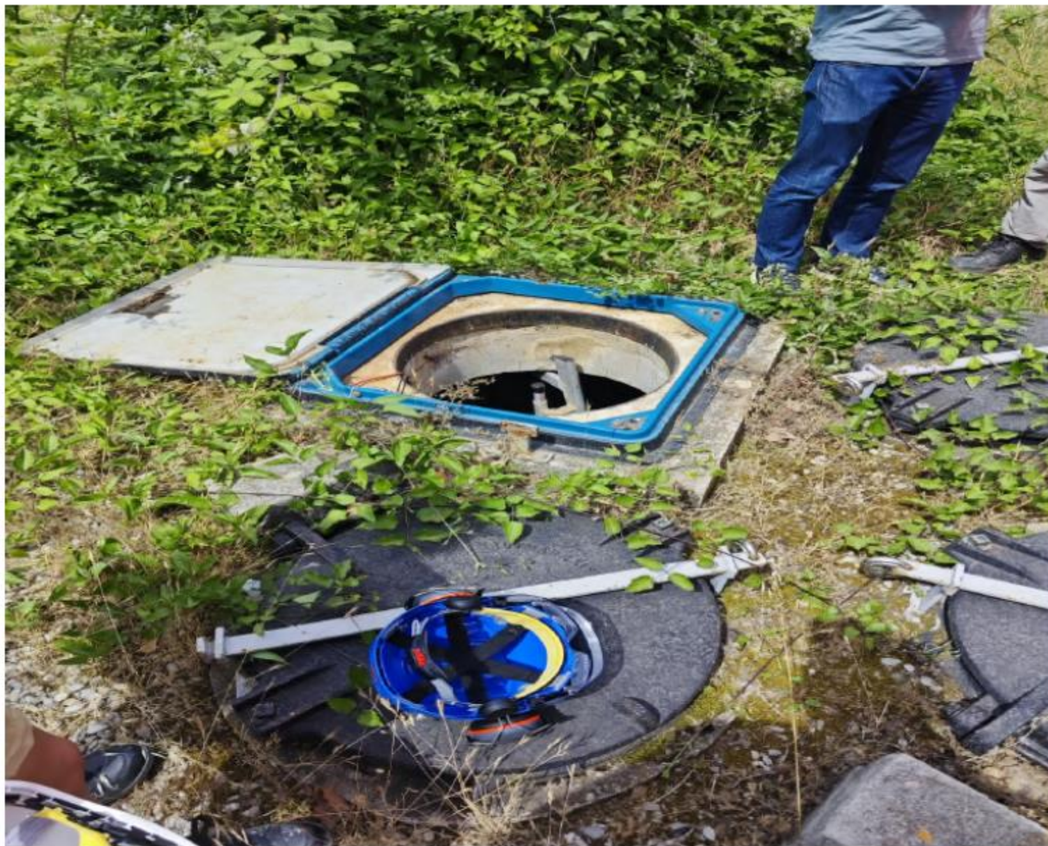
Station de pompage
